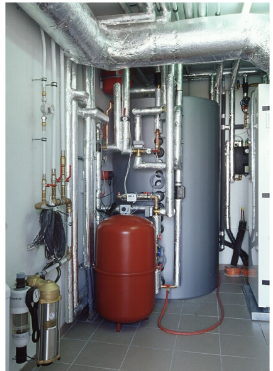
Saving energy, equipment of a passive house, May 2008, Germany Source: KfW photo archives, photographer: Thomas Klewar
