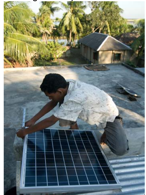
Installation of a solar home system in Bangladesh Source: KfW photo archives, photographer: Jörg Böhling
